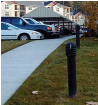
Figure 3D-21B Pathway Lighting
